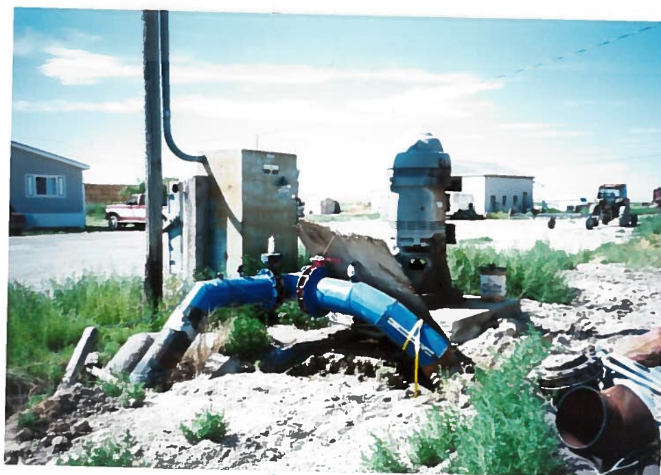
Walker Well T 10S, R 24E, Sec. 28 SWSESE 43-02359
