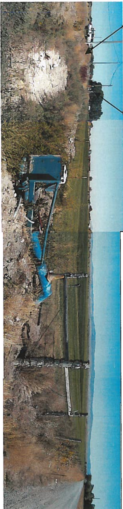
This photo set was taken at the southwest corner of the place of use and you are looking north on the left to east on the right. The pumping system in the foreground delivers Cassia Creek water into the mainline system to be delivered to the place of use. The well is located at the end of the pond to the left of the pickup. The well ties directly into the mainline and does not dump into the pond. Cassia Creek water comes in from the left at the north end of the pond.
