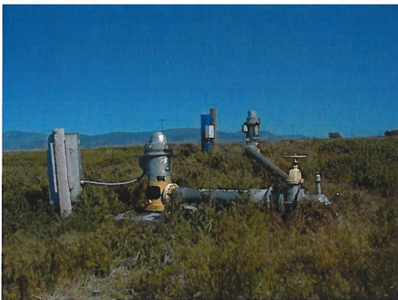
Figure 2. Backup irrigation well looking northeasterly.
