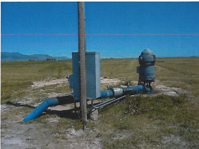
Figure 8. Main LDS irrigation pump. Looking north at POU.
