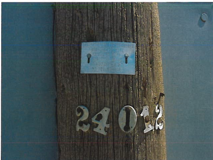
Figure 7. Power Pole for the main LDS Church Farm pump. Site tag A0007912.
