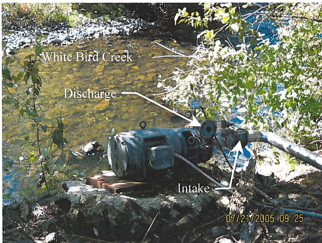
Photo 1: POD. Facing south. Intake line flips over into creek when in use.
