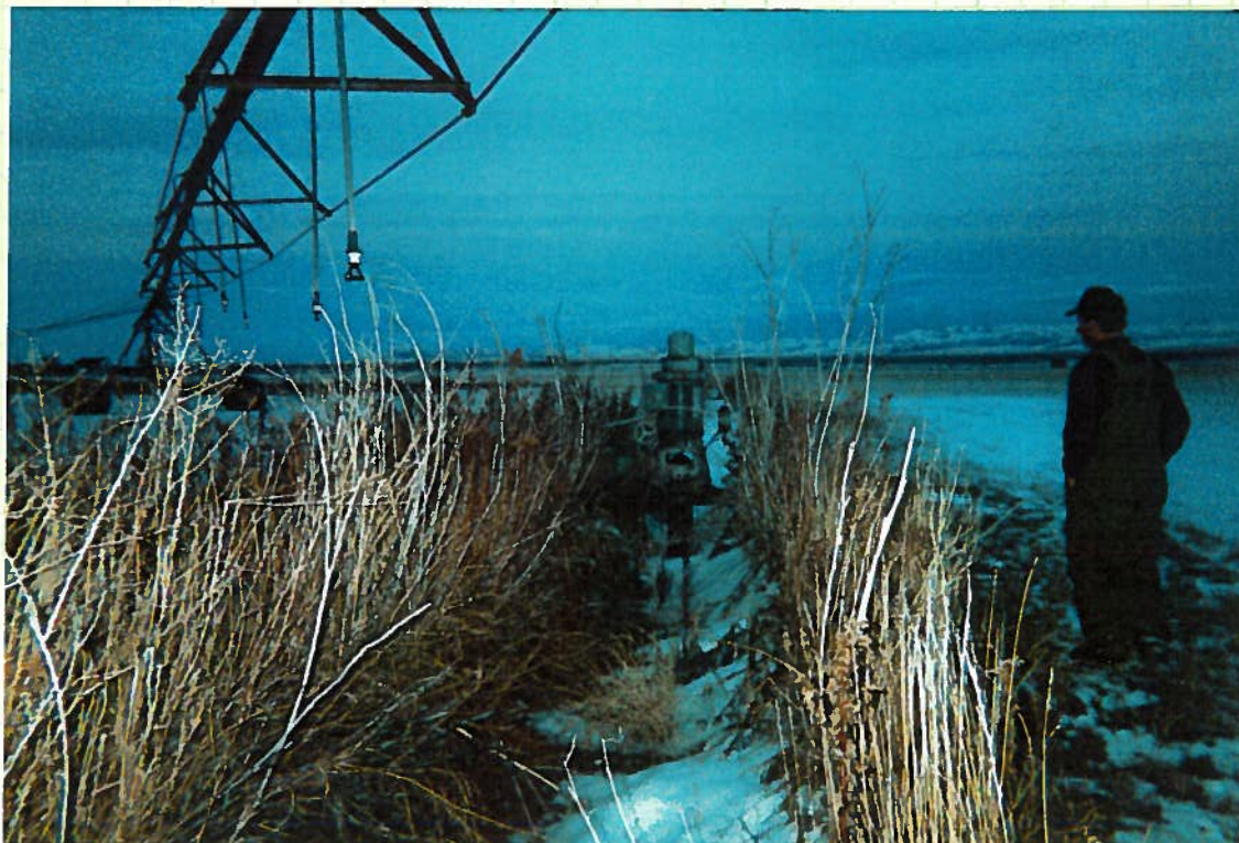
PHOTO 7. LOOKING NE AT THE WELL BOOSTER PUMP AT THE CENTER PIVOT
