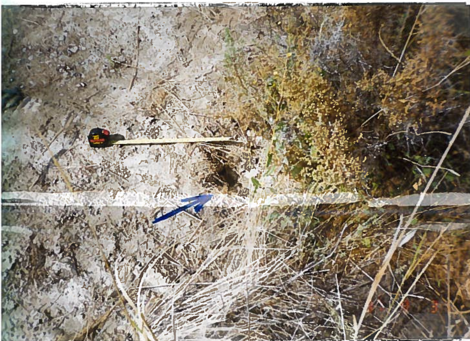
VIEW OF DOWNSTREAM END OF SAME CULVERT SHOWN IN PHOTO ABOVE. NOTE THAT CULVERT IS PLUGGED WITH DIRT, DEBRIS, AND VEGETATION, AND THAT CULVERT OPENING (INDICATED BY ARROW) IS ONLY A FEW INCHES WIDE.
