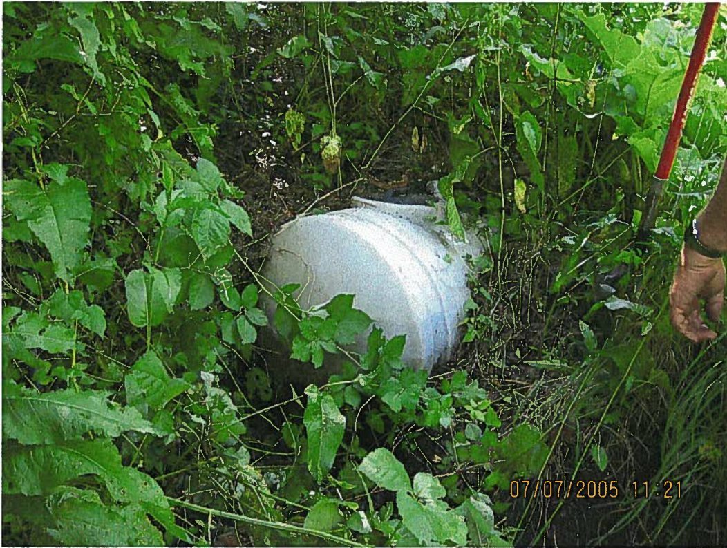
Photo 3: POD. Collection tank for the house.
