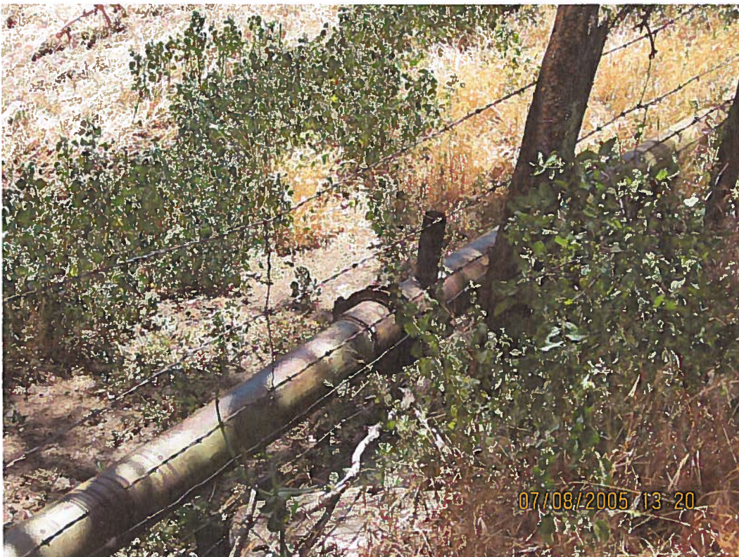
Photo 6: Sprinkler main line on eastern most pasture along Salmon River.
