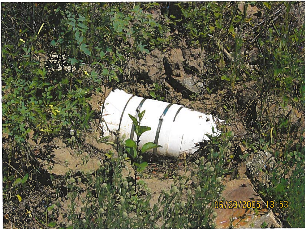
Photo 3: Ten inch PVC conveyance pipe.
