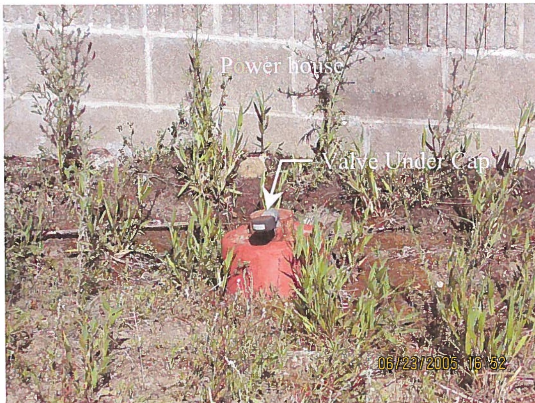
Photo 6: Valve separating irrigation water from powerhouse water.
