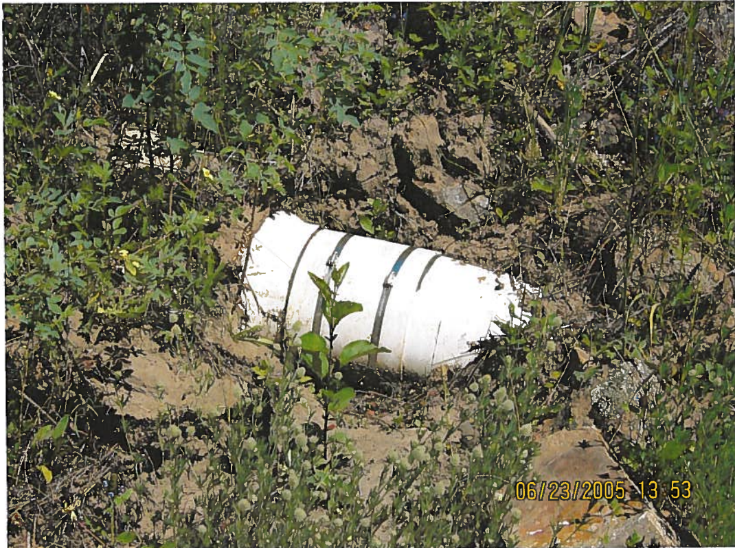
Photo 3: Ten inch PVC conveyance pipe.
