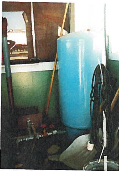
#2 Pressure tank located inside well house.
