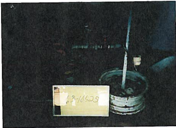
#1 Pump located inside small well house.
