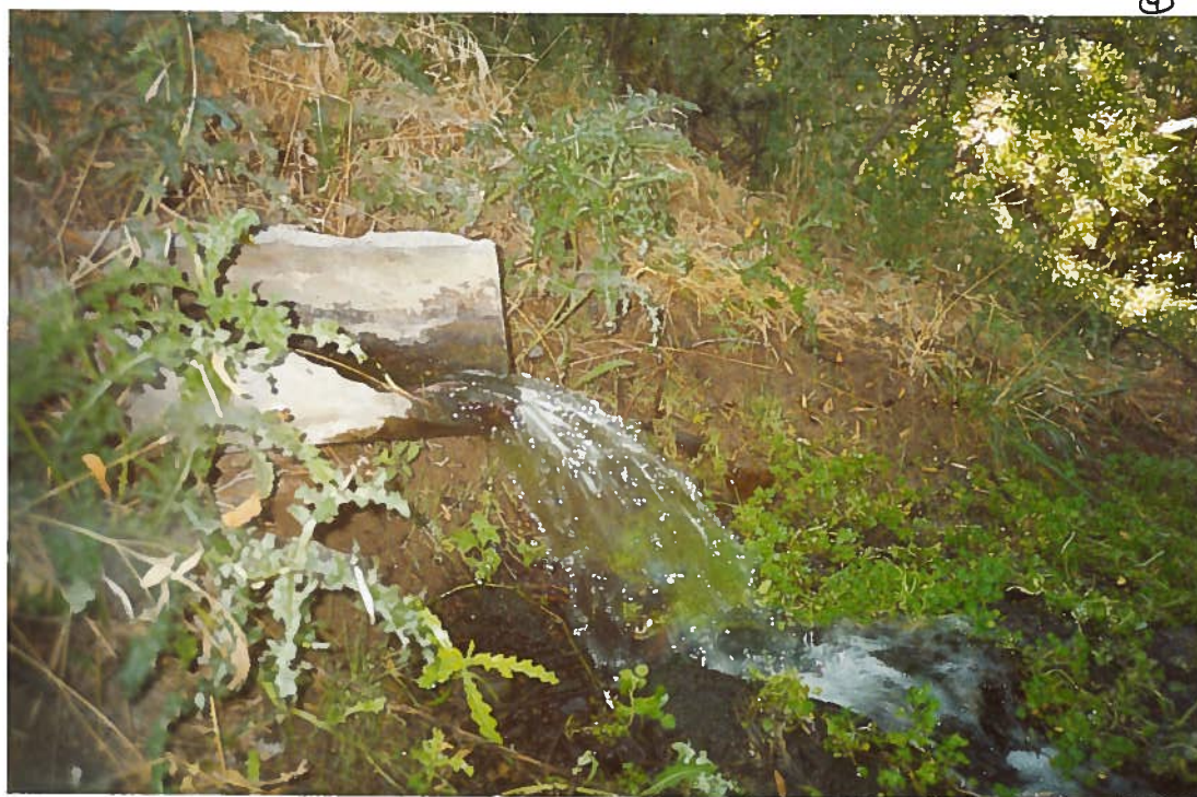
④ Discharge pipe from Spring No. 1 into channel below Spring No. 2. Flow measured at .016 cfs (Av. 7.23 gpm)
