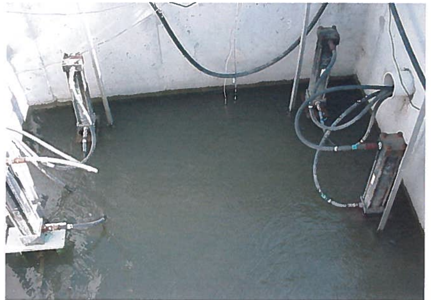
Catch basin from Diversion - 4 hydraulic valves - Each valve to different pump
