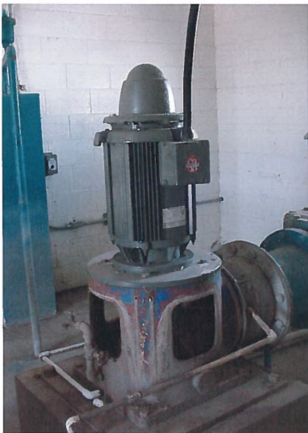
↑ Silt Water Pump Station NWSE, S19, 4N, 3W Only used on "green" pivots in SW1/4, S19 25 HP - 3 phase
