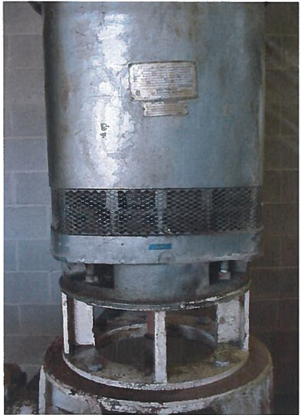
↓ Pump #1 - 100 HP 2 phase
