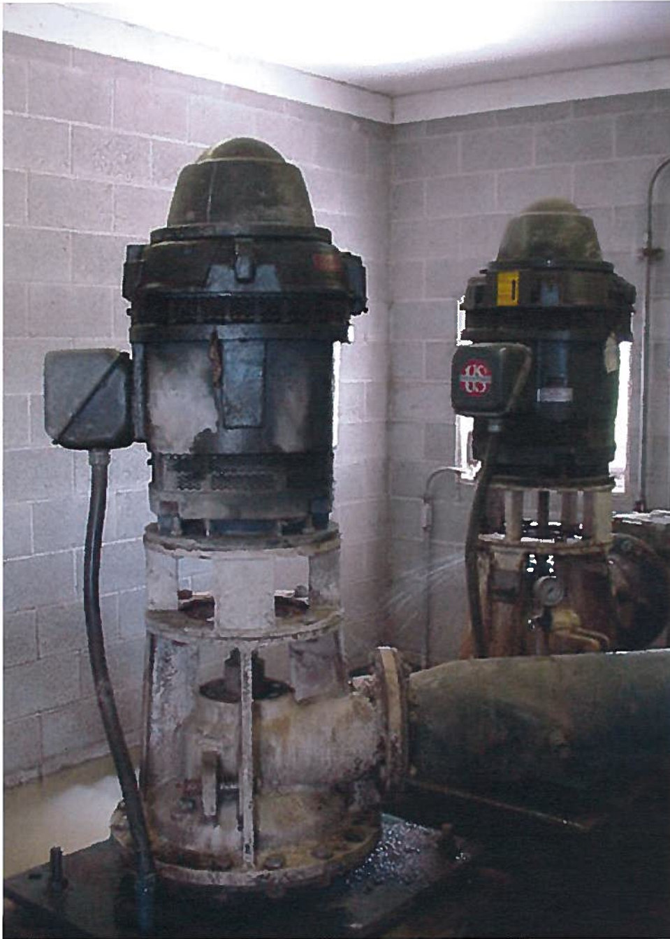
⑤ Pumps # 3 & #4 - 10" pipeline to center pivot
