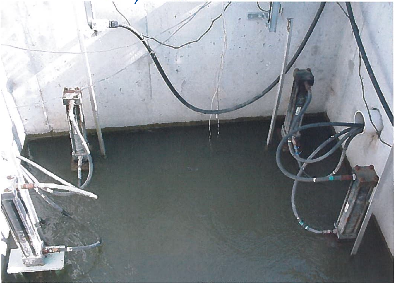
Catch Basin from Diversion - 4 hydraulic valves-
