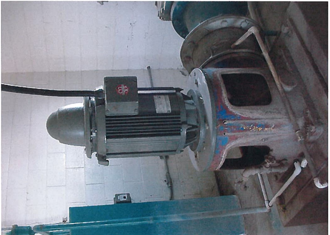
Silt Water Pump Station - NWSE, S19 - used on "green" divots in SW 1/4 S19 2540-3 phase
