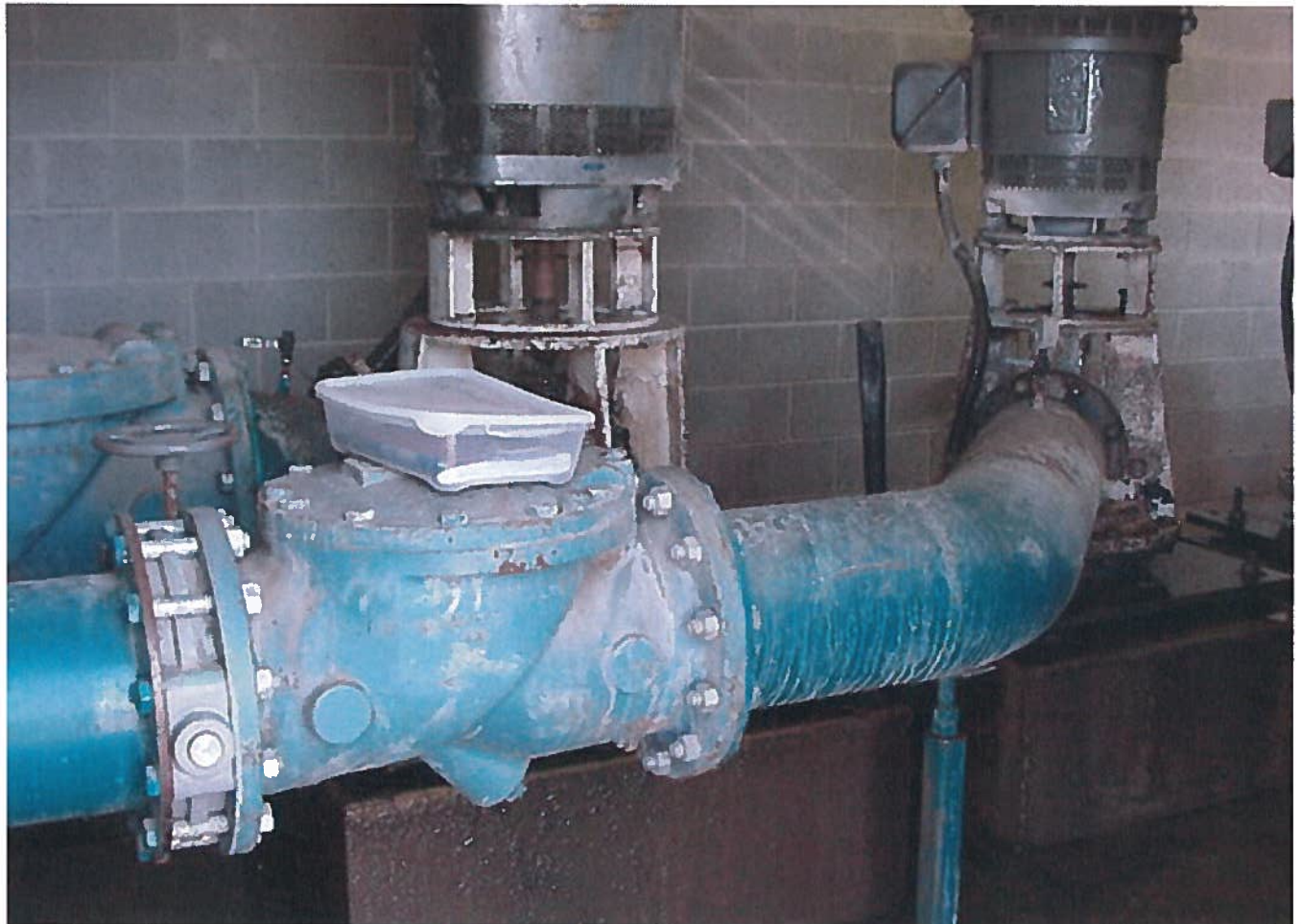
Pump #1 & #2 with 10" pipeline to center pivots ③
