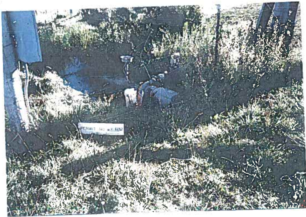
"Pump" pump Looking North- west
