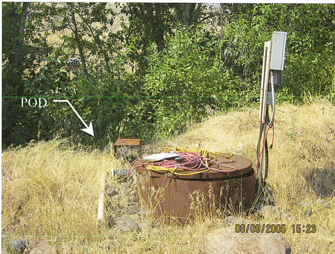
Photo 1: Looking northwest at well with submersible pump.
