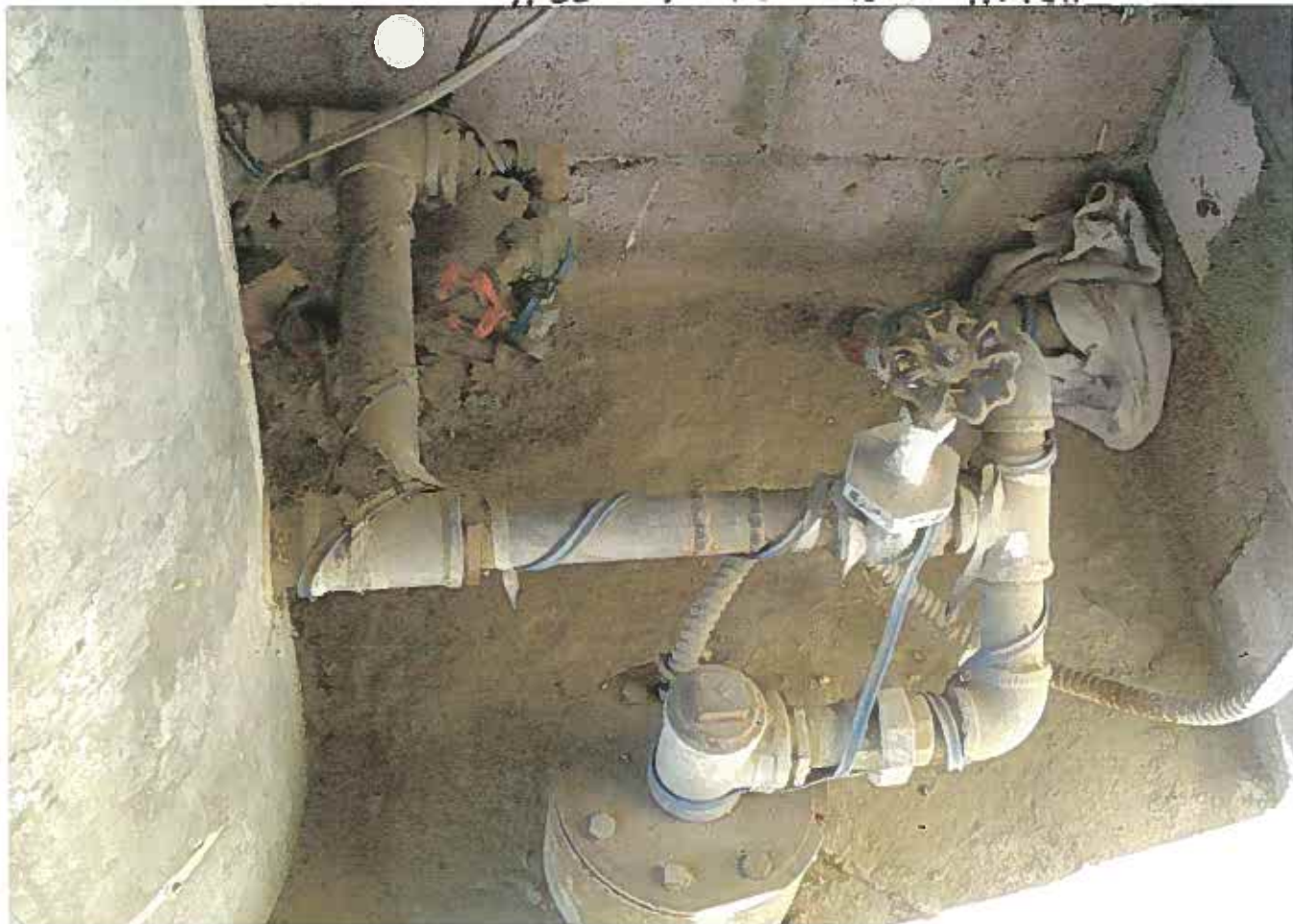
Pic:#1 Well + piping
