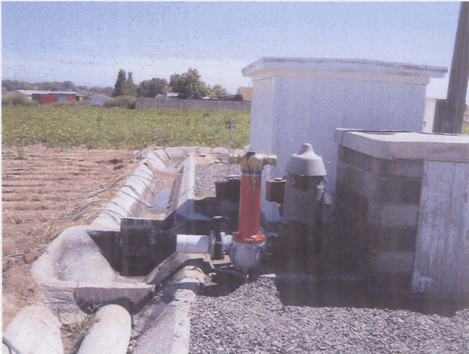
Looking East: This is the original location of the POD for 63-27331. Pump SN: 72098. 10HP, 3 phase, 60 cycles. The licensing FE shows a 5 HP pump and is identified as having a pump number of T21017. This is a different pump than was originally licensed
