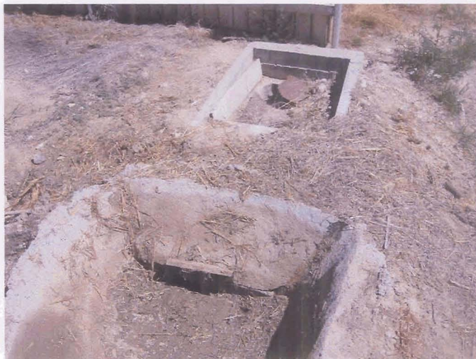
Looking East at the north control box that would historically allow water from the North well to flow under the road to the southside of the road.
