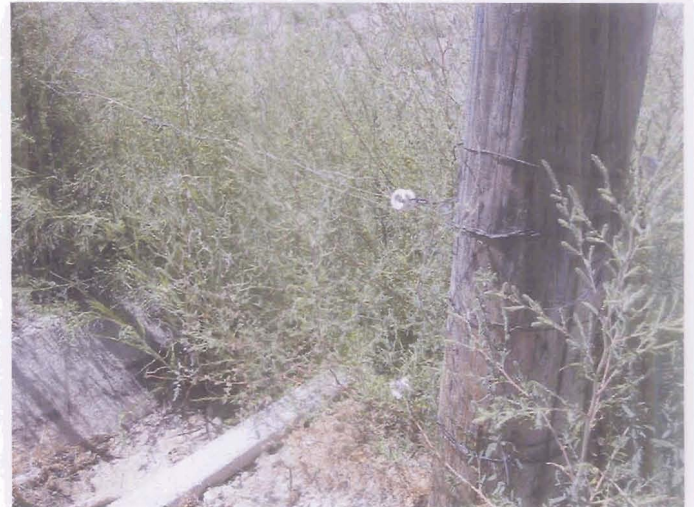
Looking West: This shows the ditch running under the fence that acts as the boundary b/w the Ashworth and Southside property. This shows that Water could get to both properties in the past.
