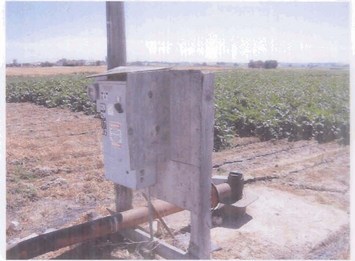
Looking SE at the current POD for 63-2733C. This appears to be an accomplished change in POD, but I cannot verify when the well was drilled.
