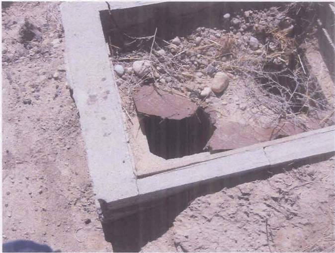
This is the control box on the south side of the highway that after the water came under the road, would allow the water right holder to divert the water to the east or west to irrigate ground on the south side of the road.
