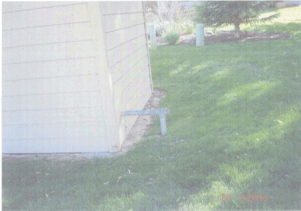
4in Pipe leaving Pump House
