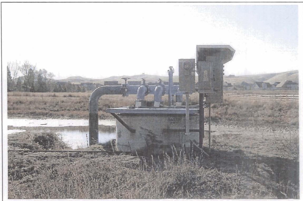
Photo 6: Distribution pond with re-lift water pumps. Piped into pressurized sprinkler irrigation system. View is to south in the SWNE, S31, T05N, R02E.
