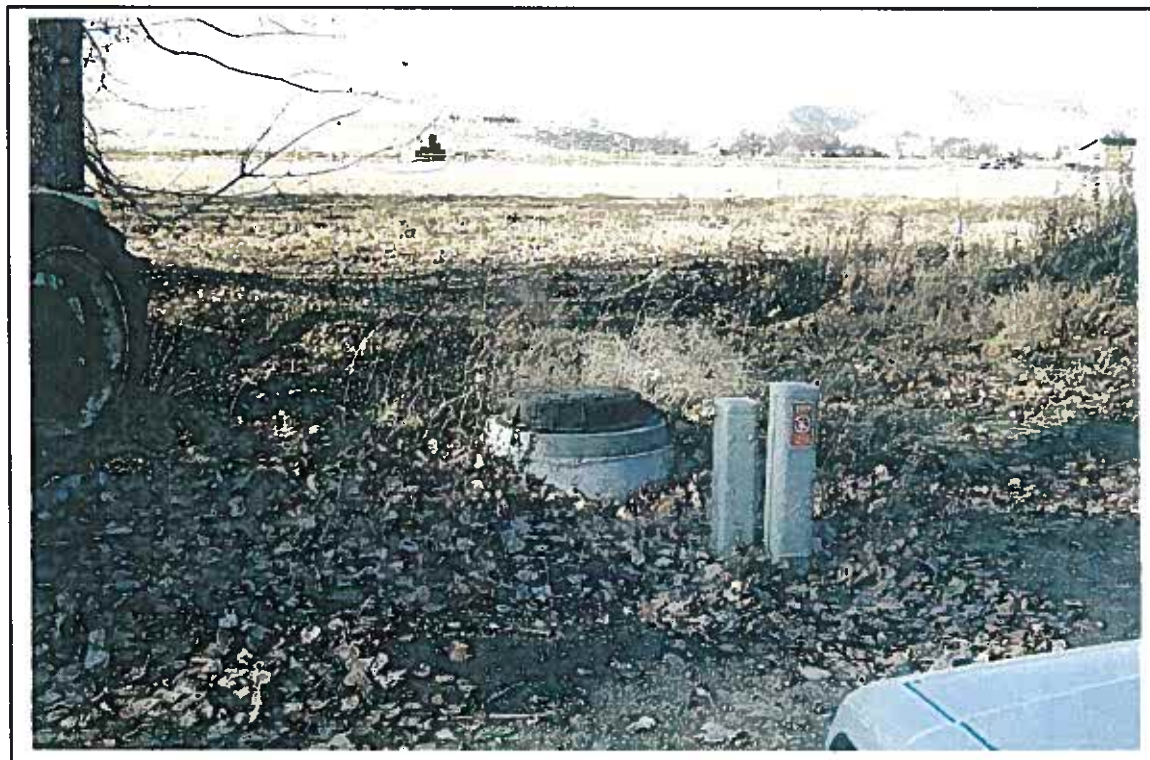
Photo 4: Manhole with gravity flow from Dry Creek on West side under McFarland Creek road.
