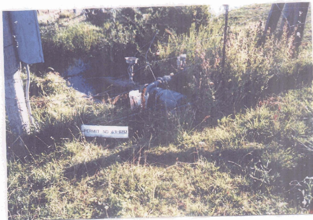
"Booster" pump Looking North- east
