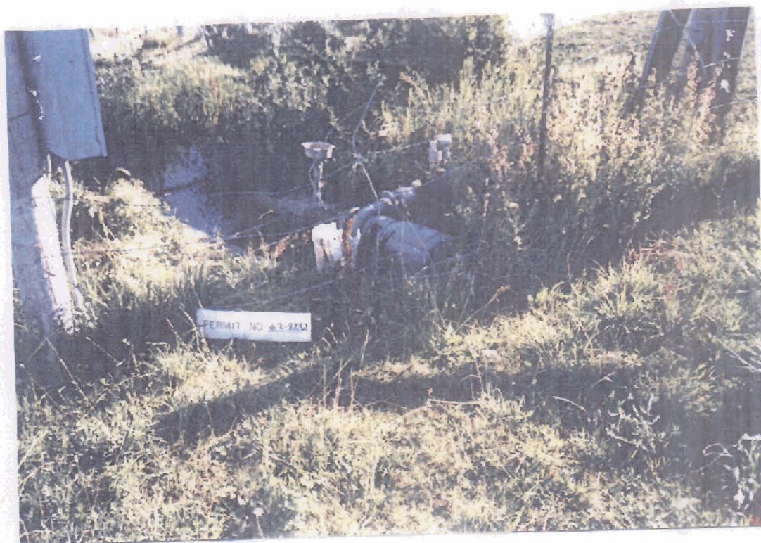
"Booster" pump Looking North- east
