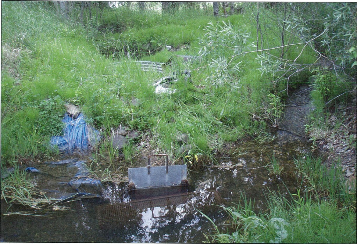
Photo 4 (6-25-09) - Facility for collection of seepage from the dam. This feature exists on the east side of the embankment. At the time, the rate of flow in the ditch (right) was estimated ~20-25 gpm.
