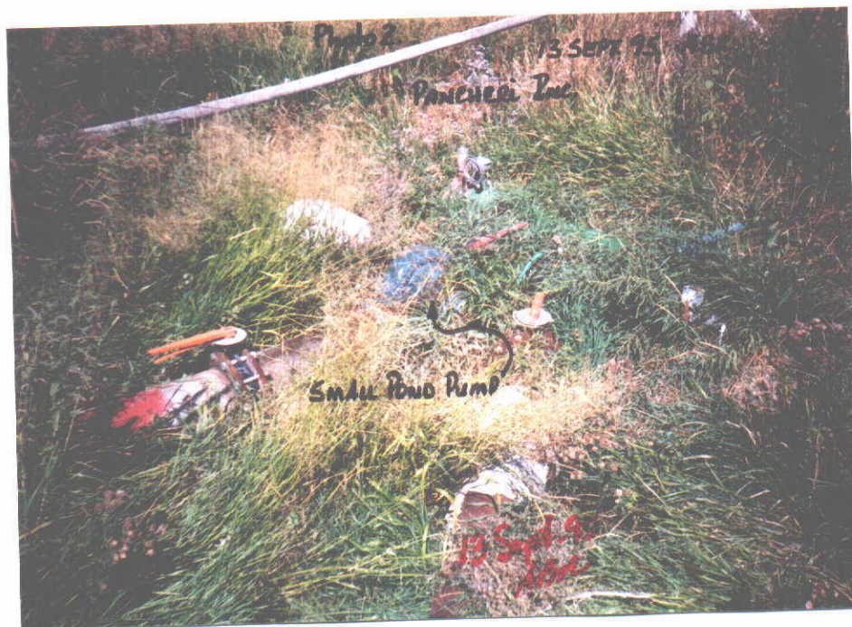
Photo 2. Shows Small Pond Pump AND (THROUGH THE WEEDS) SOME OF THE PIPING WHICH CAN, CONNECT ALL PUMPS AND THE WELL TO ALL THE DISTRIBUTION SYSTEM.
