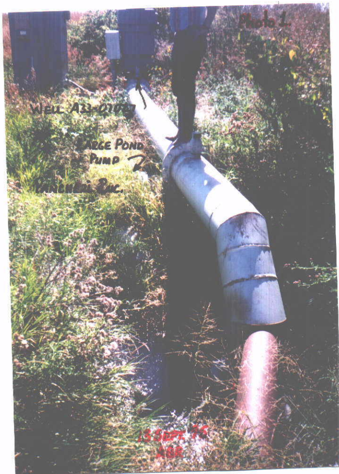
PANCHERI, INC. Photo 1. Shows Well 33-07027 IN BACKGROUND. PERSON STANDING ON PIPELINE IS ERNIE CARLSEN - UNDER WHERE HE IS STANDING IS THE LARGE POND PUMP. SEE SKETCH.
