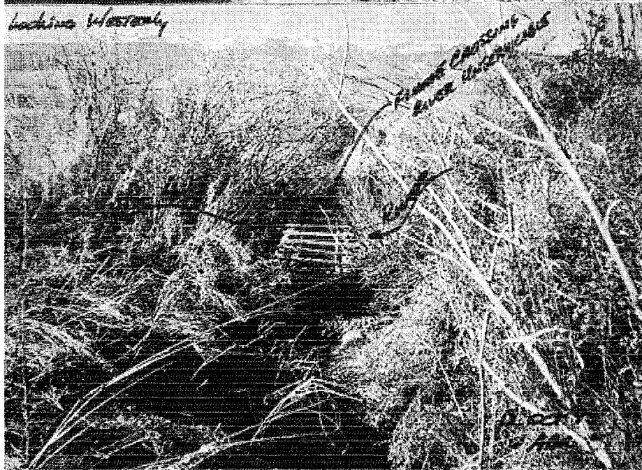
Photo 2. OLD UNDERSIZEABLE FLUME CROSSING LITTLE LOST RIVER (HIDDEN IN UNDERGROWTH - FLOWING RIGHT TO LEFT). THIS FLUME CARRIED BADGER CREEK AND/OR LITTLE LOST RIVER EXCHANGE WATER TO THE WEST SIDE OF LITTLE LOST RIVER. SEE DEER CREEK CLAIM A33-10119. NO LONGER USED.
