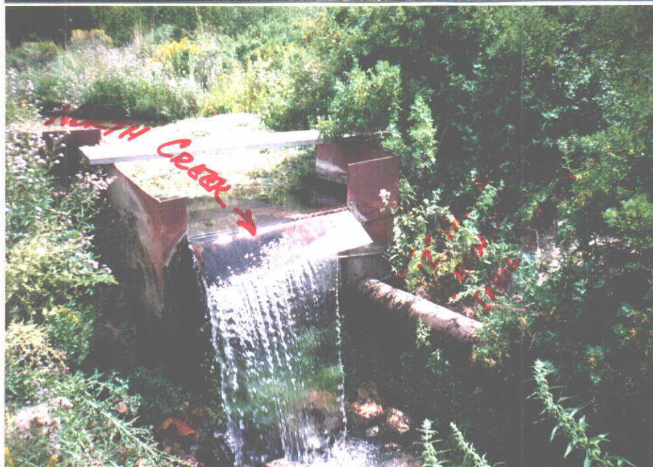
Photo 2. POINT OF DIVERSION FOR AND 33-02023 DAVID WAYMIRE'S A33-02012. SHOWS 12 inch STEEL MAINLINE AS BEGINNING OF IRRIGATION SYSTEM.
