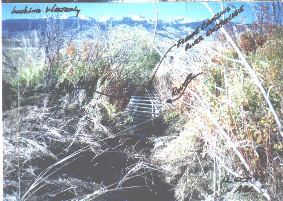
Photo 2. OLD UNSERVICEABLE FLUME CROSSING LITTLE LOST RIVER (HIDDEN IN UNDERGROWTH - FLOWING RIGHT TO LEFT). THIS FLUME CARRIED BADGER CREEK AND/OR LITTLE LOST RIVER EXCHANGE WATER TO THE WEST SIDE OF LITTLE LOST RIVER. SEE DEER CR CLAIM A33-10119. NO LONGER USED.
