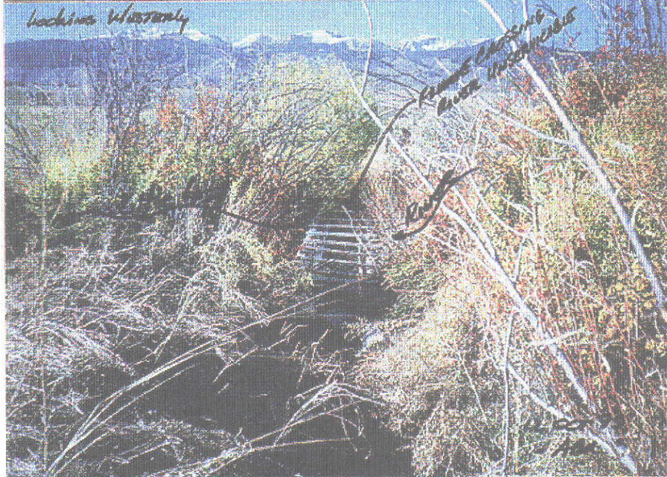
Photo 2. OLD UNSETTLEABLE FLUME CROSSING LITTLE LOST RIVER (HIDDEN IN UNDERGROWTH - FLOWING RIGHT TO LEFT). THIS FLUME CARRIED BADGER CREEK AND/OR LITTLE LOST RIVER EXCHANGE WATER TO THE WEST SIDE OF LITTLE LOST RIVER. SEE DEER CREEK CLAIM A33-10119. NO LONGER USED.
