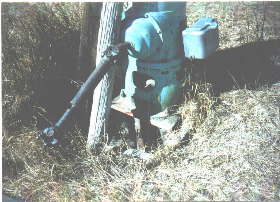
Fig. 2 - Close-up of PTO-powered pump showing inadequate well seal.
