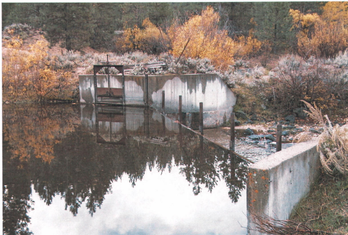
Photo 2: Same as above. View is from West side of Smith Creek to East. Screw Head gate.
