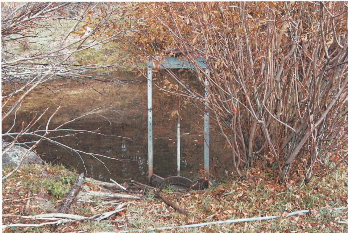
Photo 2: Screw head gate on east bank.
