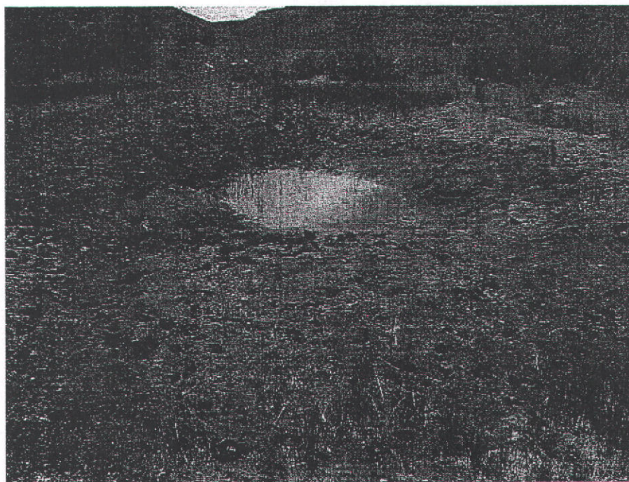
Minimal storage capacity due to partially washed out dam.
