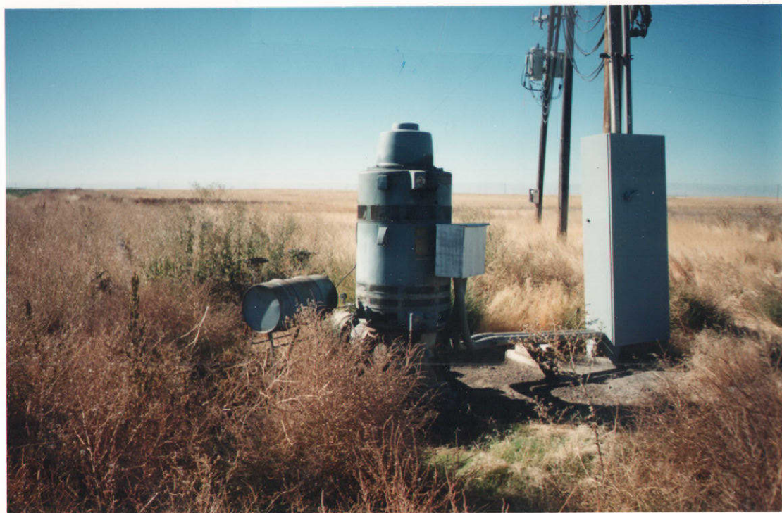
⊥ Photo #1 10-8-96 Looking SW FROM the NE NW NW corner of Sec 19 showing Pump #1
