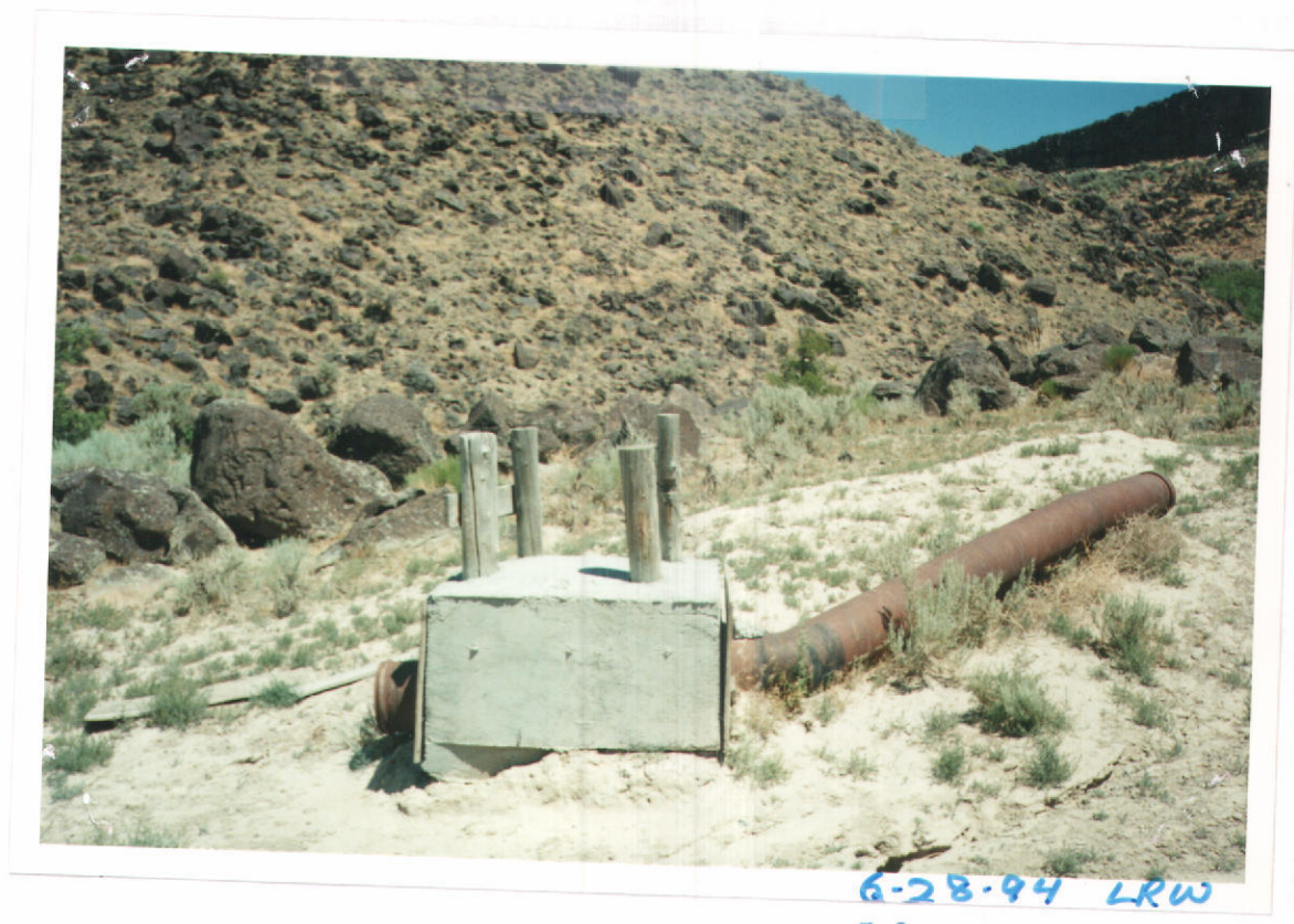
Second control box, 12" pipeline
