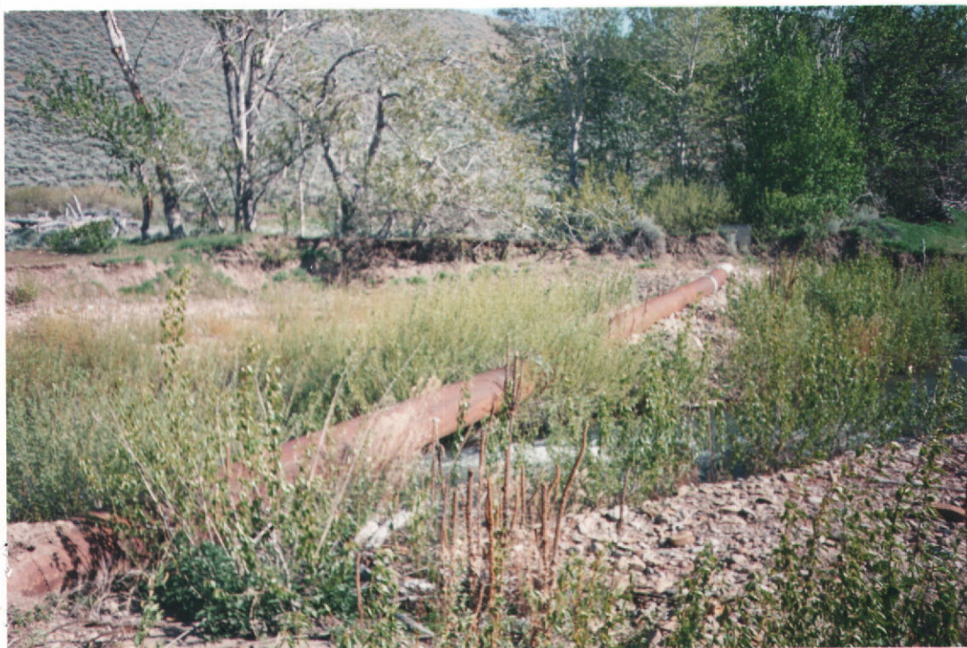
PICTURE #2: This photo shows pipeline from the gate valve of above photo, this pipeline is for the East Side ditches. View is to the North West on East side of Cold Springs Creek.
