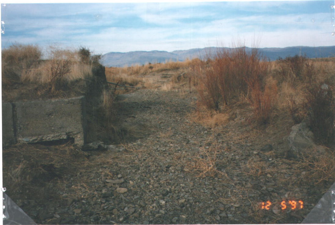
PICTURE #1, COLD SPRINGS CREEK: Follow-up FX Dec 5, 1997. Photo's by RDH. P/D no change from last photo's in 1994. View upstream, lack of maintenance for diversion, abandoned.
