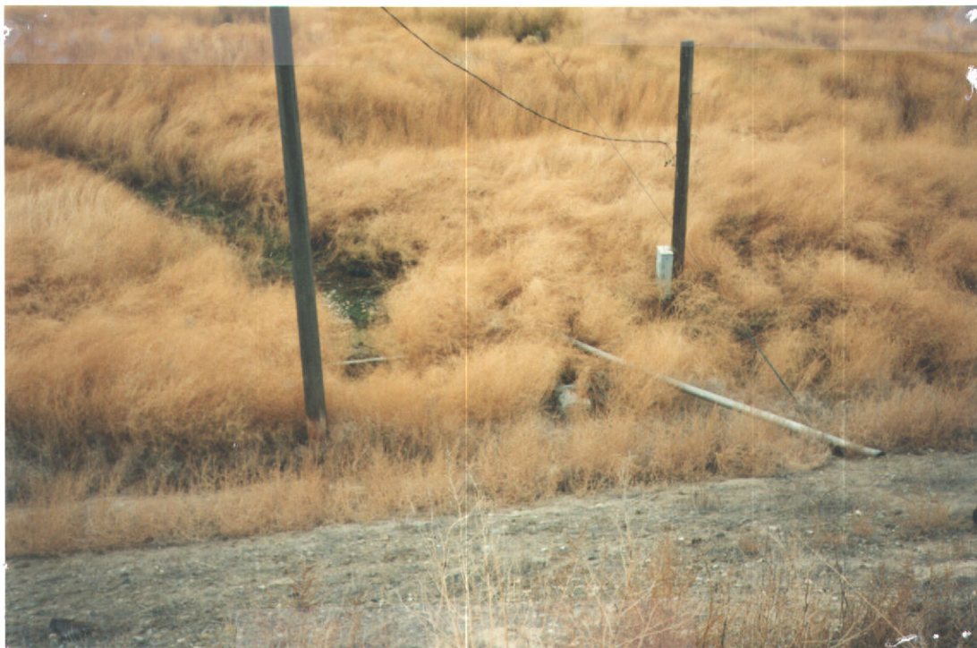
Pumping plant no. 7 75 HP Pump
