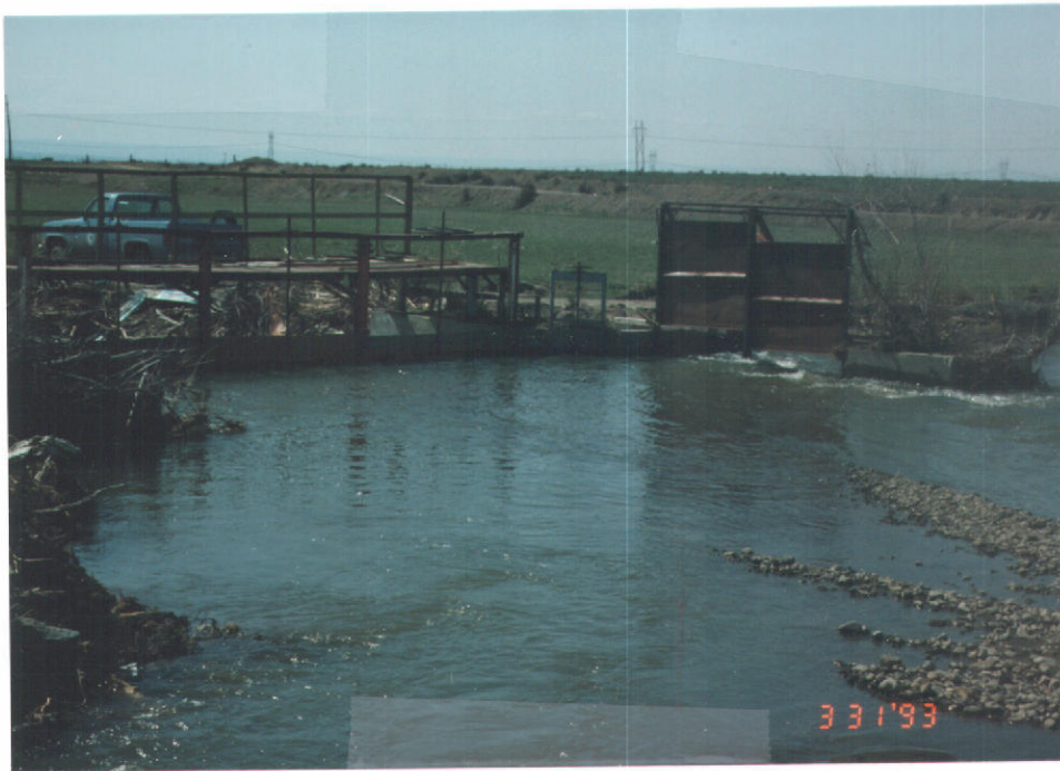
Diversion structure in Bennett Cr. at P/D
