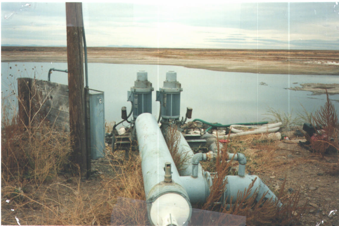
Pumping plant no. 6. 2. 100 HP pumps
