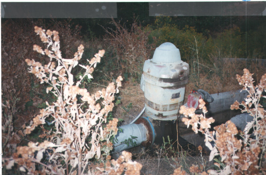
② Pump, located on south side of creek. Pipe goes under- ground and connects w/GW system.
