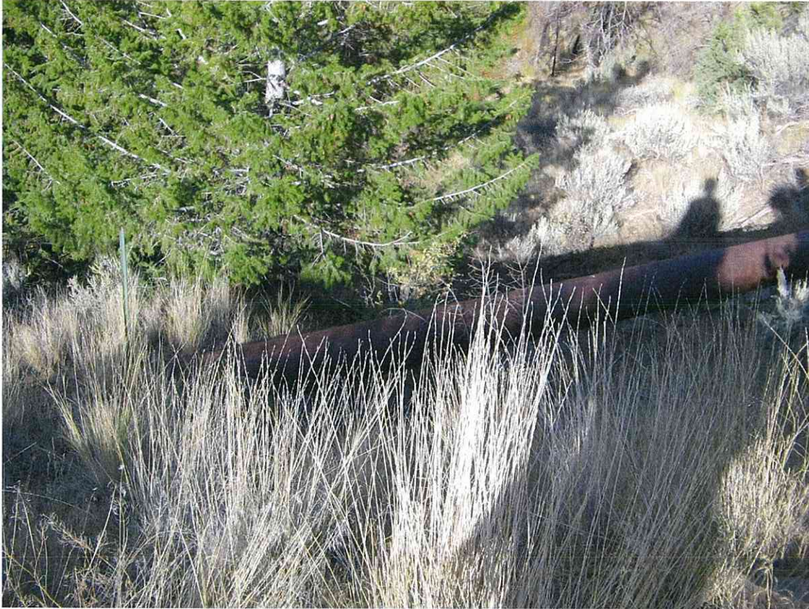
This pipe was exposed near the PVC pipe seen in the last photo. Presumably the PVC pipe has replaced corroded sections of previously installed metal pipe.
