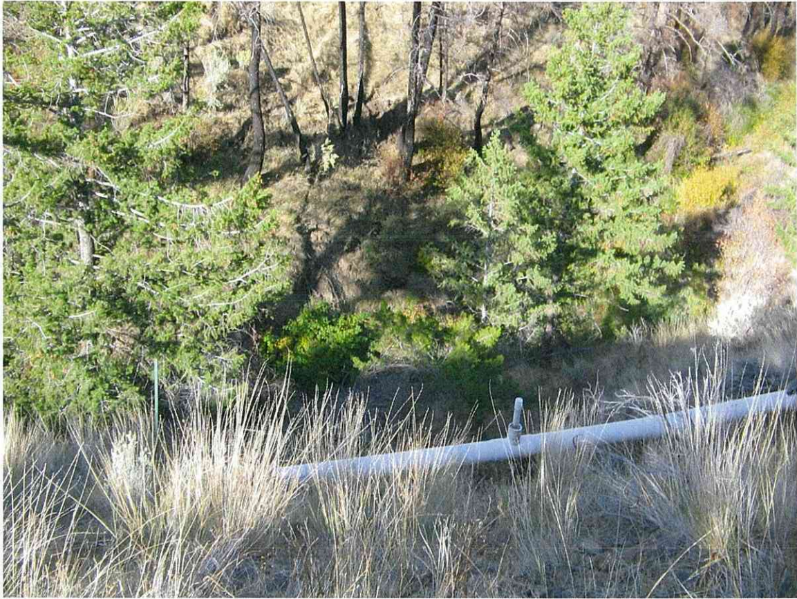
A second view of the exposed pipe. Picture taken facing southward toward the South Fork Sevenmile Creek channel.
