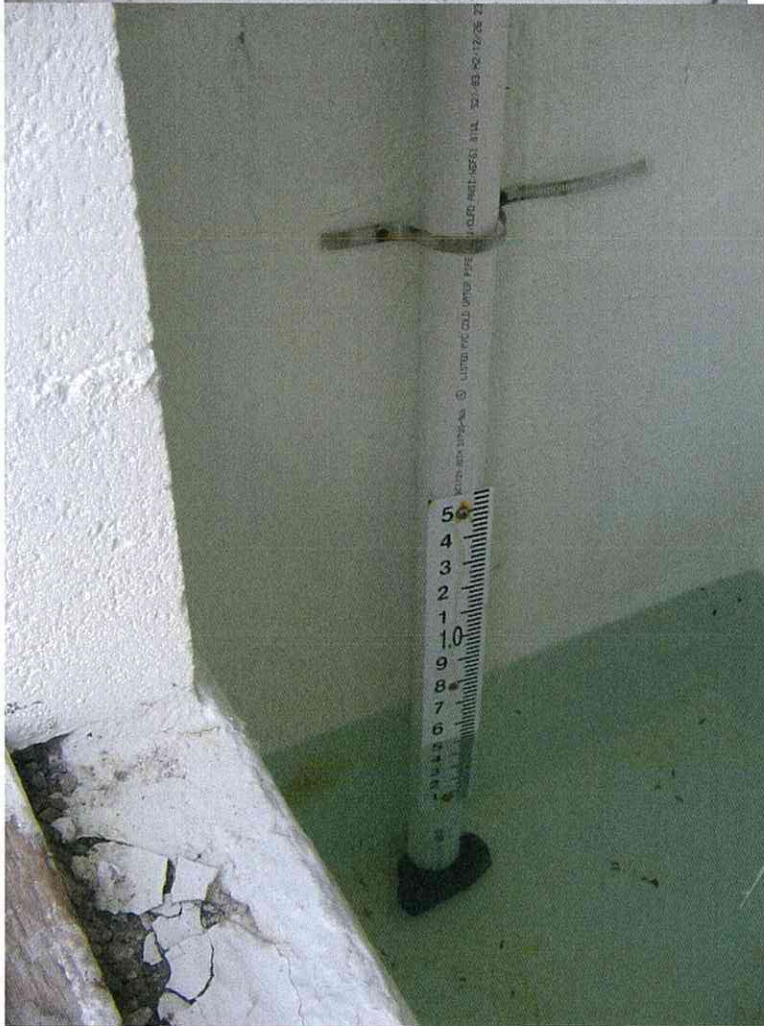
Pictures showing inside of spring box for 75-7032.
