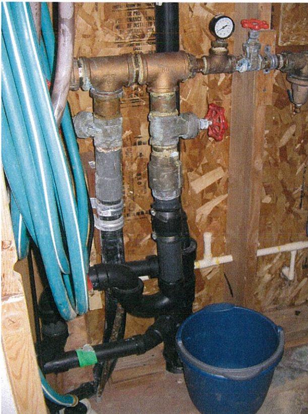
Entry point for water to the current bottling plant. According to Mr. Tacke, the gauge will read 100 psi during operation and has a reducer on it (extreme right) because of the extreme pressure in the system. The springs are approximately 200 feet in elevation above the level of the bottling plant.
