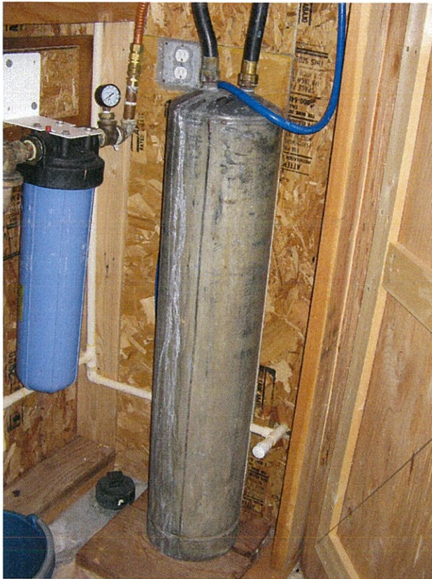
Filter for water entering the bottling plant.
