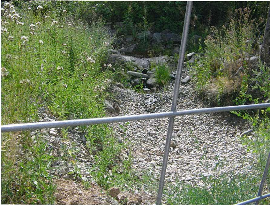
Photo shows Arrowhead Water Dist's gravel filtration for its domestic right. The pipe from the Chipps Creek diversion can be seen in the center background. The pipe dumps water into this gravel "trough," where it is collected in the 2-inch pipe that then goes to serve the homes.
