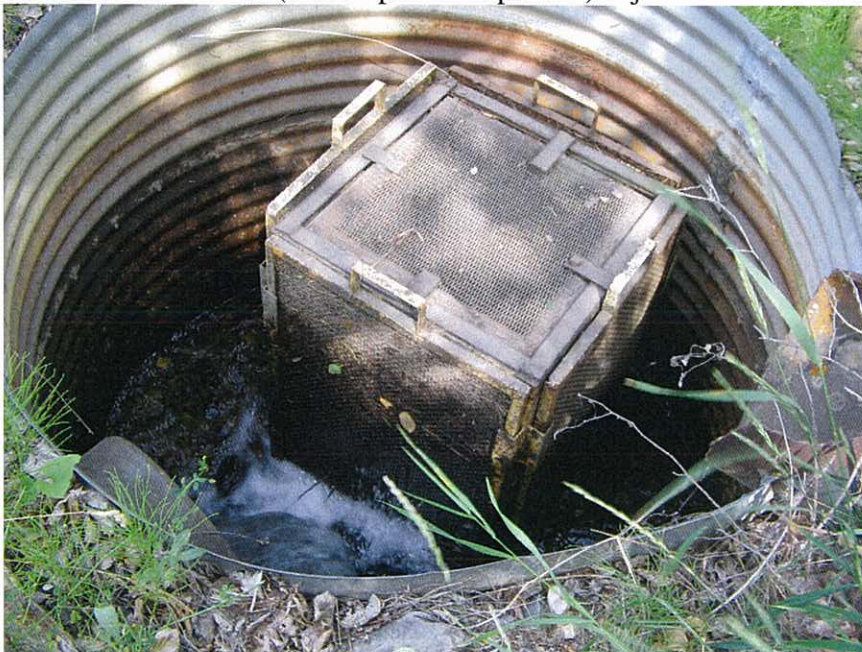
Photo showing Pollard Creek ditch/reservoir water dumping into Arrowhead's piped irrigation system.
