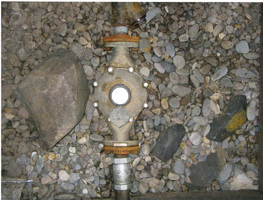
Photo showing Arrowhead's gage for its domestic right from Chipps Creek. Per Gary Lysinger, member of Arrowhead Water Dist, the watermaster told him this usually carries between 30 and 40 gpm. There is a 2-inch pipe going into and coming out of this gage.
