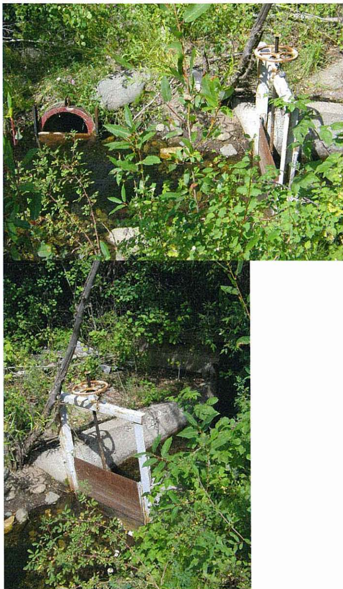
These photos show where Arrowhead measures its irrigation right from Pollard Creek. The headgate is to the right of the picture. The left of the picture shows a culvert used for overflow. The overflow runs back into Pollard Creek.
