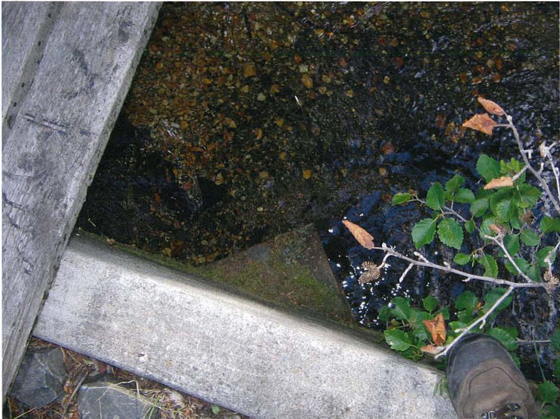
Photo from above looking down at City of Salmon Chipps Creek diversion. Pipe is approximately 12 inches. This pipe goes underground and its contents dump into Pollard Creek just above the City's Pollard Creek diversion.
