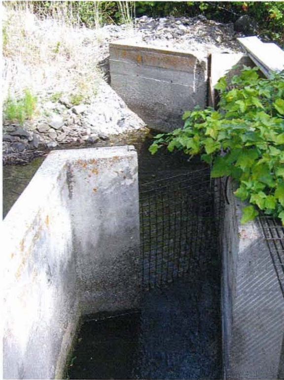
A look at the interior of the City of Salmon Pollard Creek diversion. The actual point of diversion is the wire mesh visible in the right-center of the picture. Water is diverted through this screen and flows around the corner into a pipe (shown next picture).
