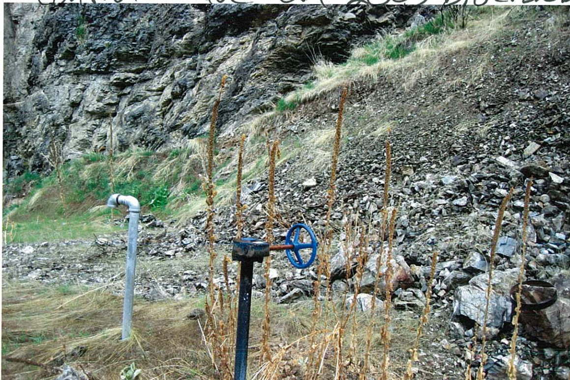
Control Valve on 2003 Diversion
