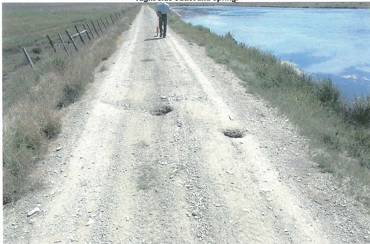
Holes in crest.
