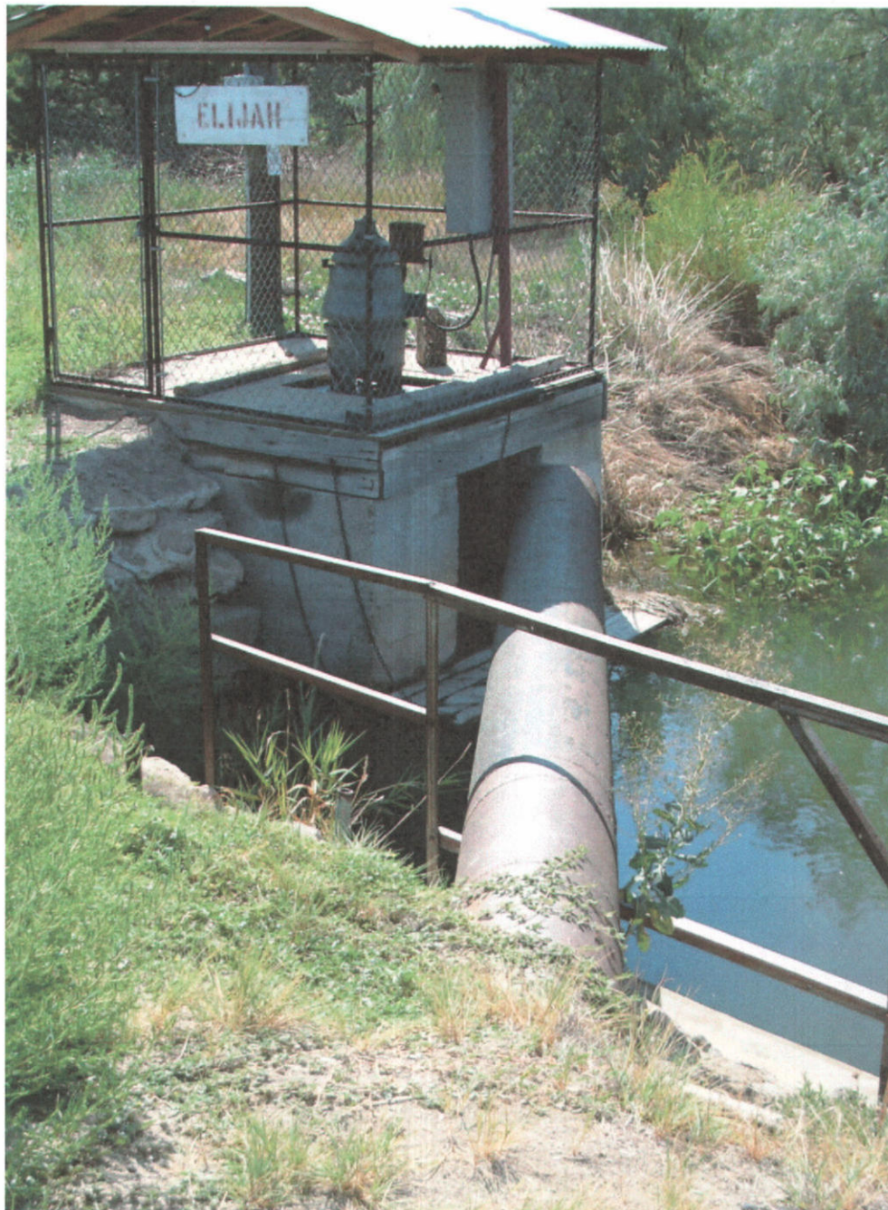
Elijah Drain Pump and Discharge Pipe
