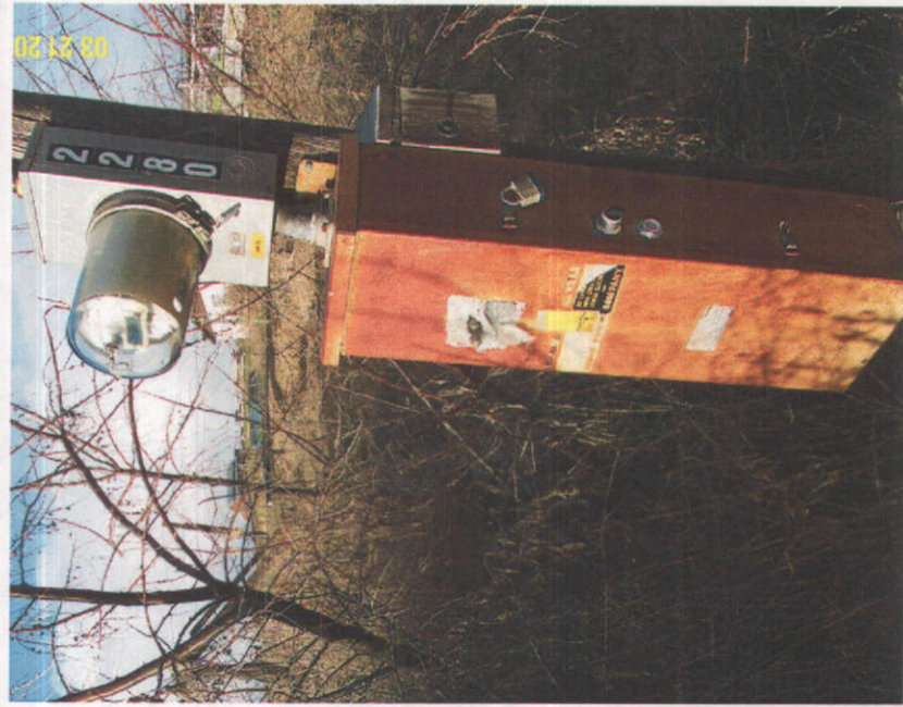
Armenta Meter & Panel
