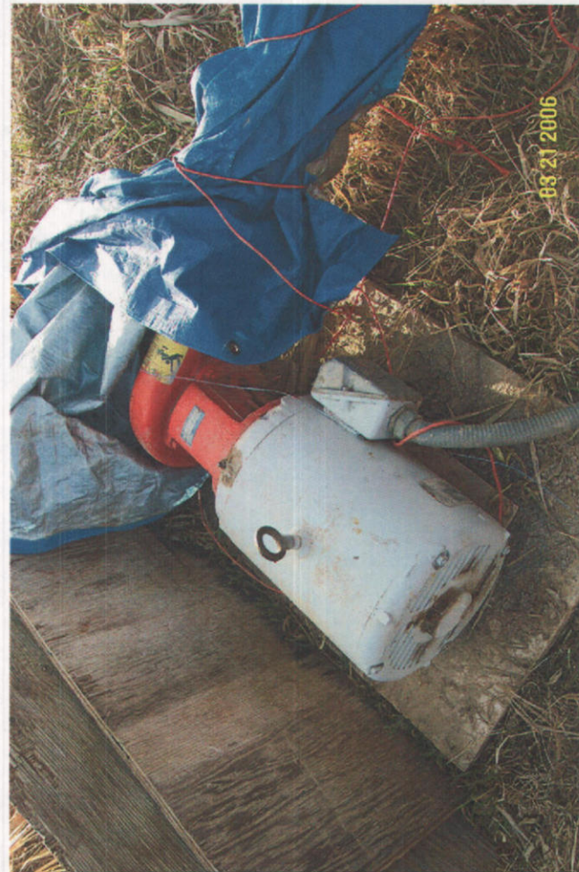
Armenta Pump 20 HP Centrifugal
